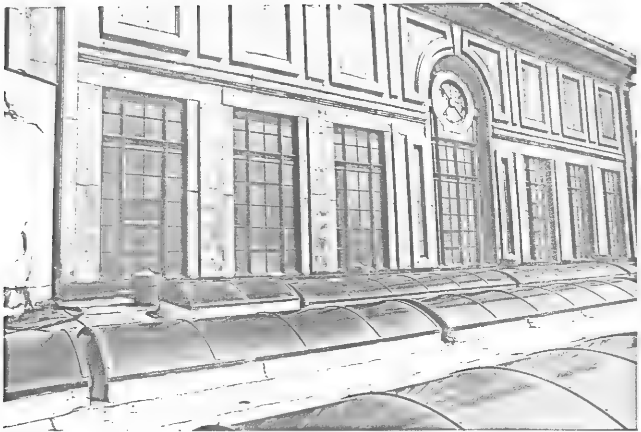
Western facade of terminal, viewed from roof of train concourse, showing plastic "bubble" type of skylight installed to replace glass block skylights removed in phase one of N.J. Transit's rehabilitation programme.
